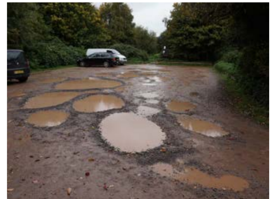
Photograph 13: Pot holes at Bersted Brooks LNR car park.
